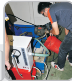
10 Adding new coolant/ water into tank for normal water level.
